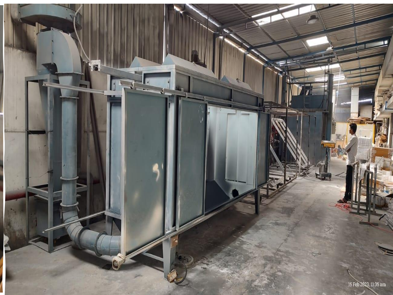
Powder-Coating & Paint Unit
